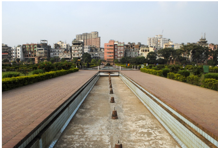
Figure 7 Broken structure, No maintenance (Source: author)
