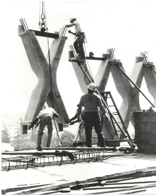
Fig. 5. Malcolm Leeland's X elements are covering the American Cement Building.
