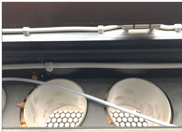
Fig. 8. View from above of two air inlets lined with short PVC stub. The slightly larger diameter cutout in the HEA240 is visible as is some sprayed-in foam insulation filling the lower cavity beneath the shape's web. The perforated closure angle is visible, but the insect screen resting directly on it is washed out in this photo by the author.
