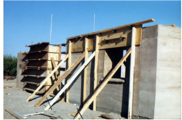
Figure 3: Second rammed earth project in construction, showing end boards and movable forms.
