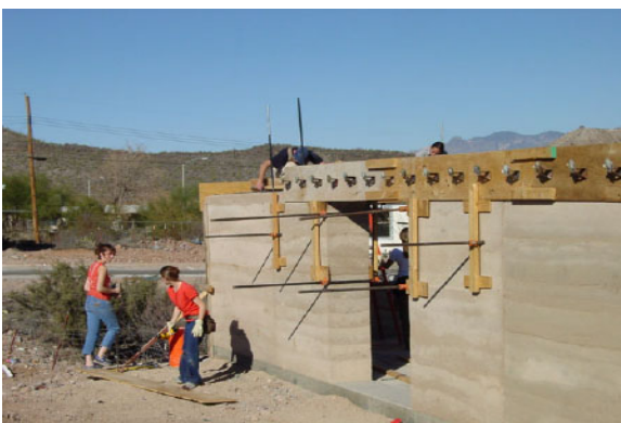
Figure 5: Third rammed earth project in construction; with pipe clamps supporting the continuous formwork for a bond beam.
