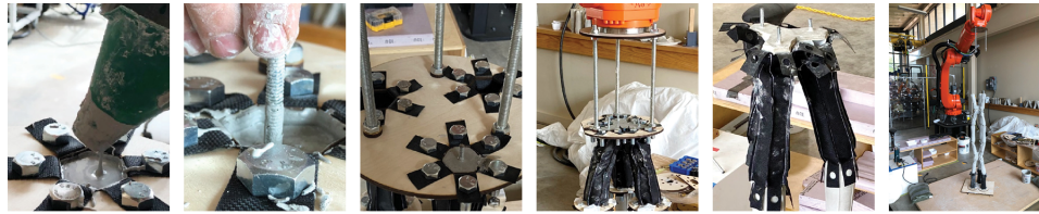
Figure 4: This image shows the process of pouring Rockite (A), placing all thread reinforcement immediately after casting (B), and leaving the material to cure (C). The bottom images represent the casting of the layers using the robotic arm (D and E) and the final column design without the base and the bottom formwork removed (F). Work by Mohammad Karkoutly. Source: (Mohammad Karkoutly 2022)
