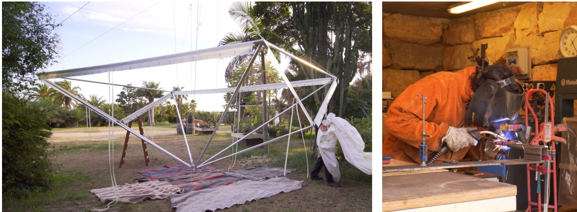
Figure 4: left: space frame mock-up, right: manual welding of steel knots. Source: (Frau Recerques Audiovisuals 2022)
