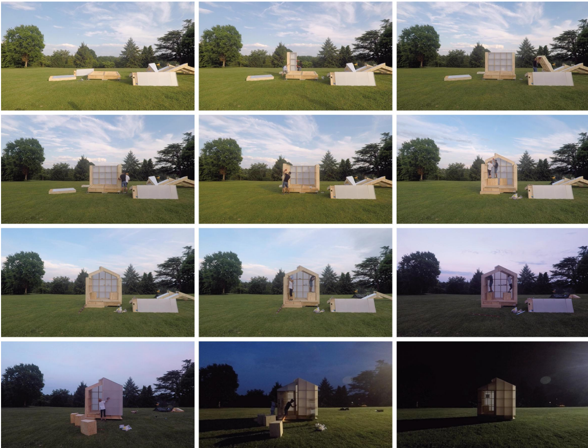
Figure 6: The integration of digital fabrication methods and construction practices enable the structure to be built in a single day. Source: Authors
